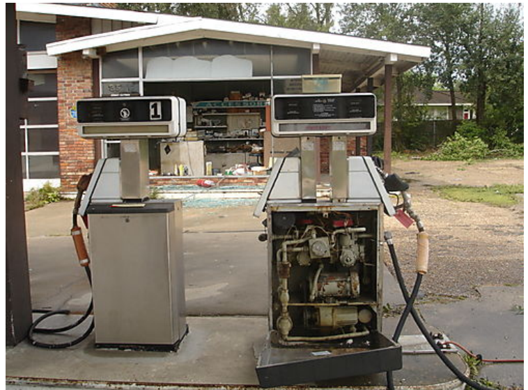
Old Gasoline Tanks and equipment at Sonny Cutrer's Shell on Government Street have been removed, but property remains an eyesore.
